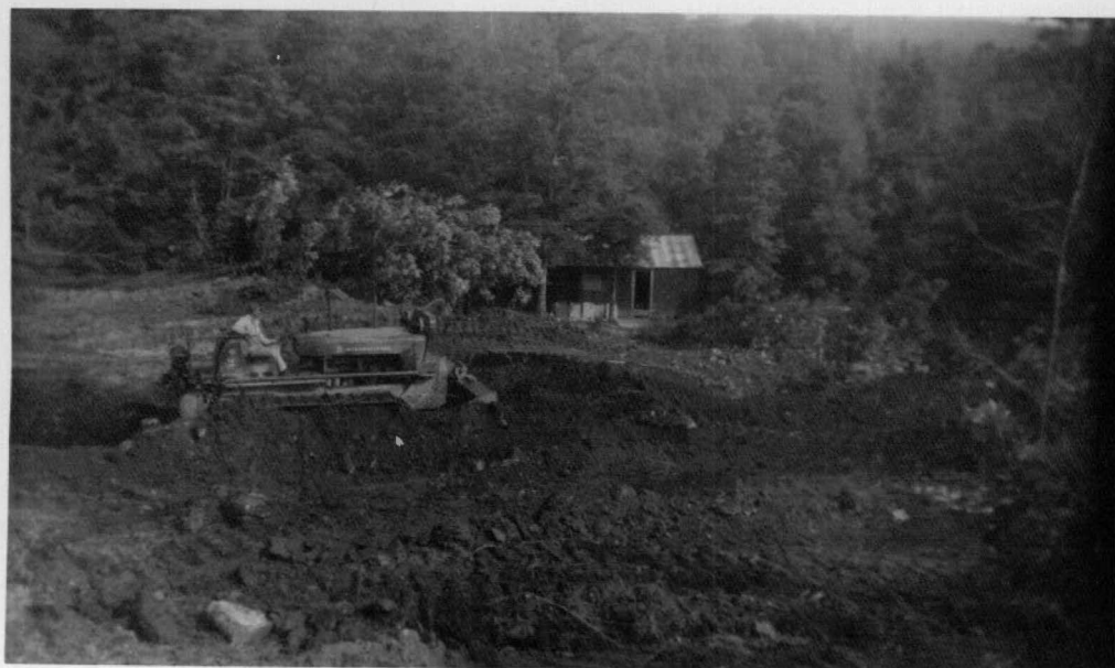
Figure 56. Clearing the surface in preparation for stripping in the western edge of the Crab Orchard Mountains area.
